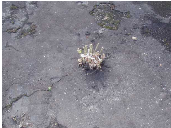
Picture 19: Destroyed tight surface, by plants
