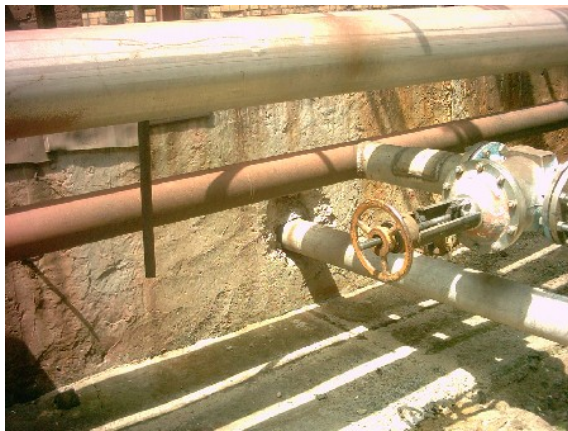
Picture 8: Pipeline in the secondary containment area
