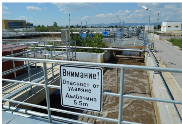
Wastewater treatment in Sofia. Photo: INTECUS GmbH
